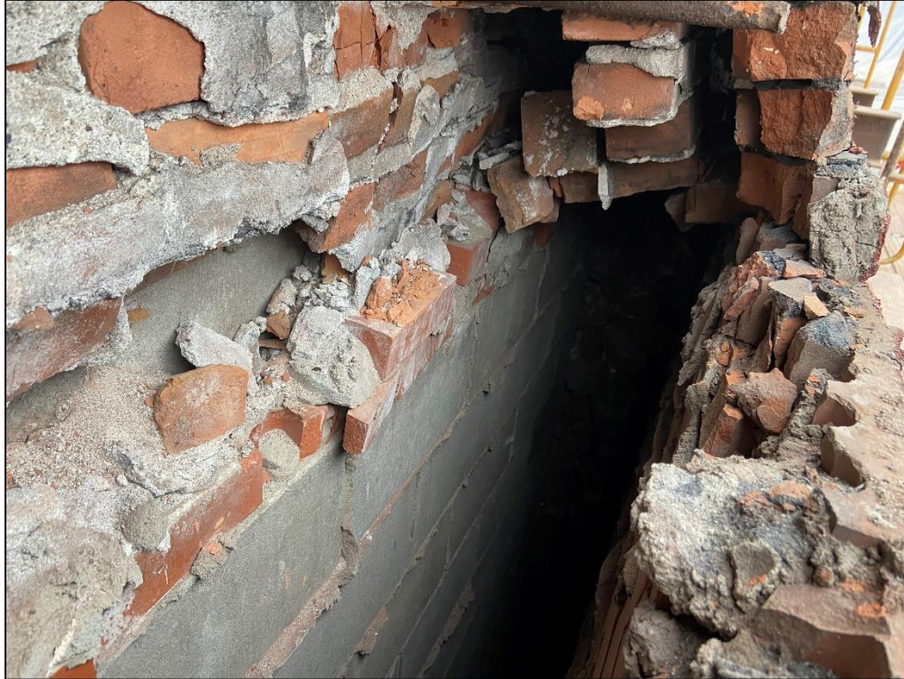
Photo 1 – Void between CMU and Clay Brick Façade
