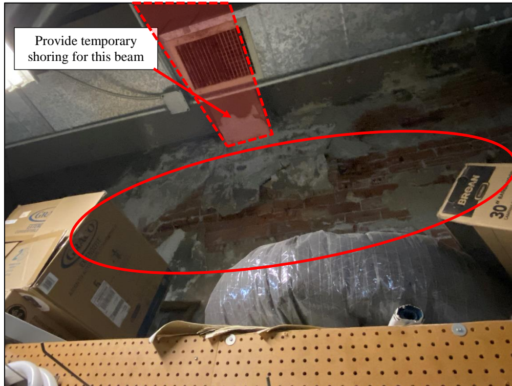
Photo 1 – Damaged Brick & Beam to Support
